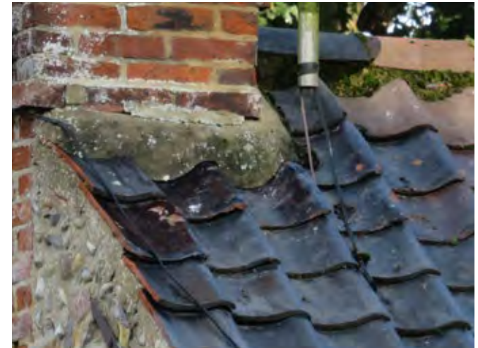
Inappropriate cementitious repairs to chimney and roof
