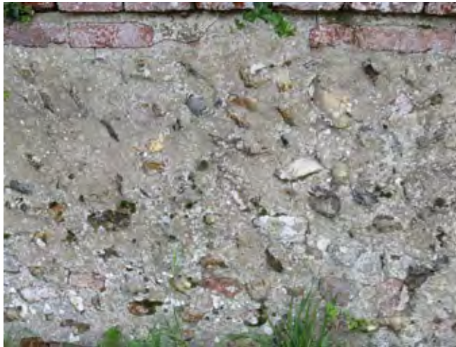
Excessive repointing to flint wall
