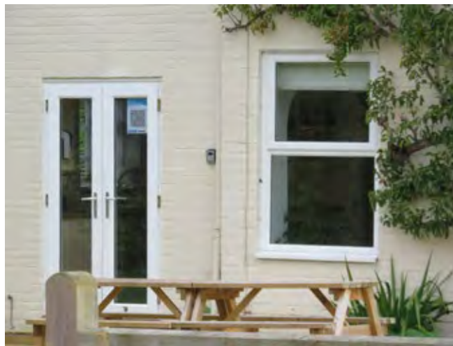
Inappropriate uPVC door and window
