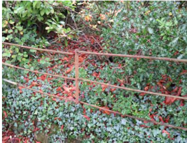
Broken and corroding railings
