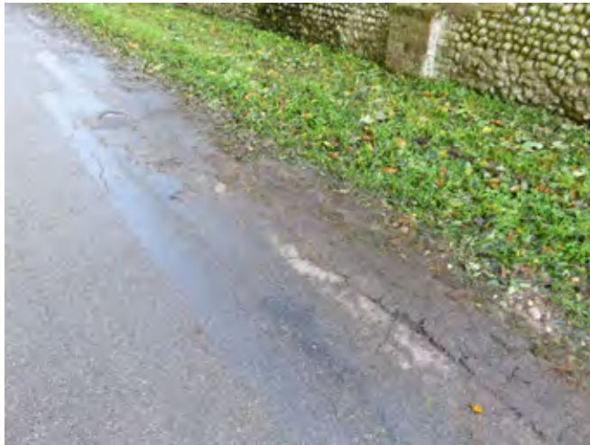
Poor road surface on The Street
