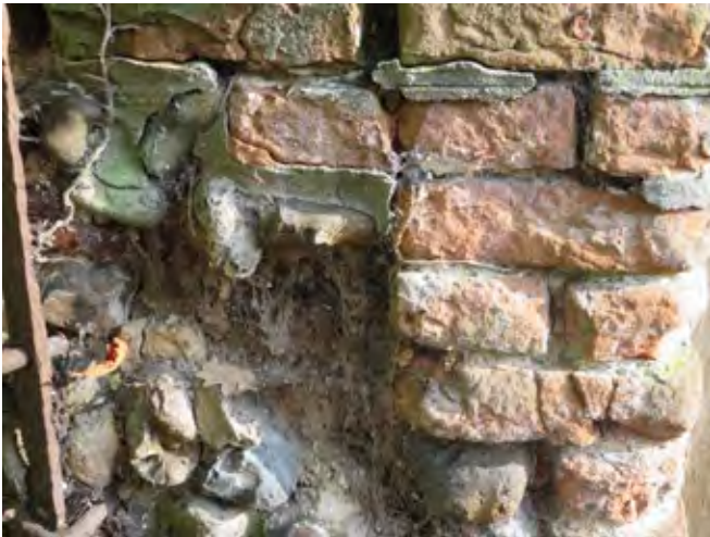
Cementitious repointing, missing flints and damaged bricks to a historic boundary wall
