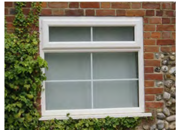
Inappropriate uPVC window
