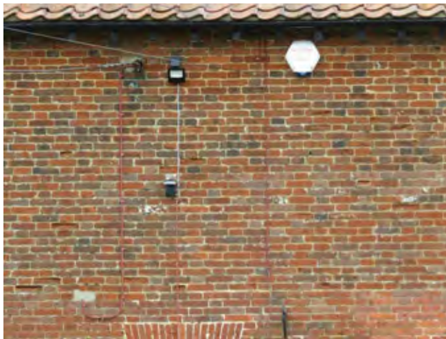
Accumulation of cables, light and security alarm
