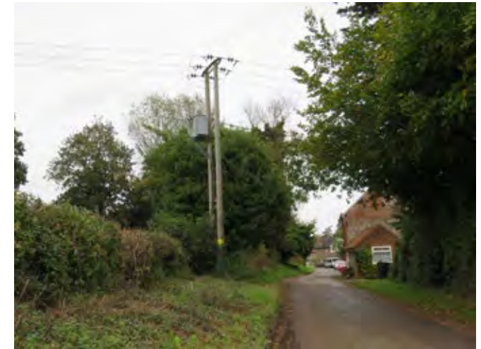
Pylon on The Street
