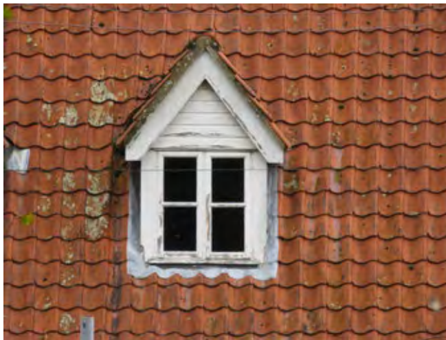
Window joinery that requires repainting
